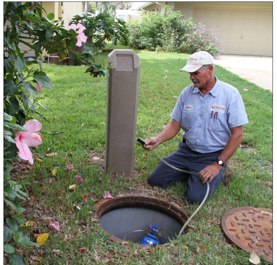
Veolia Field Supervisor John Morris checks the vacuum level in the AIRVAC system as part of a scheduled maintenance program in Crystal River. See story on Page 9.
