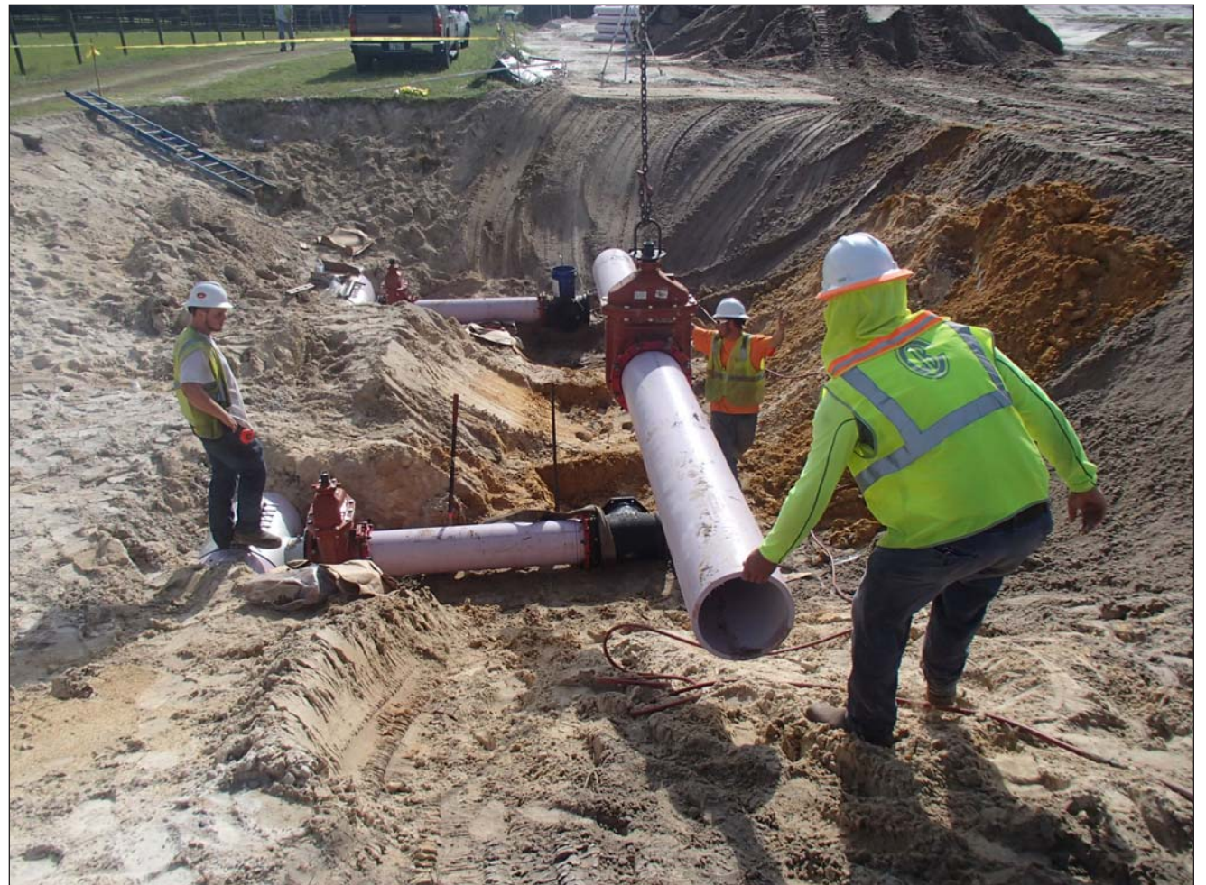
Photo courtesy of Clay County Utility Authority
