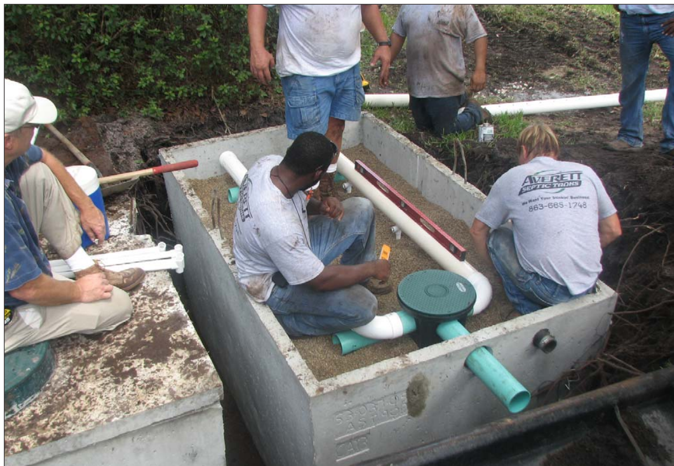
Photo courtesy of Hazen and Sawyer
