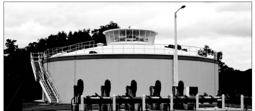
POLK COUNTY - IMPERIAL LAKES WTP 1.0 MG POTABLE WATER STORAGE TANK WITH 3800 GPM AERATOR CONSULTING ENGINEERS: JONES EDMUNDS AND ASSOCIATES, INC.
