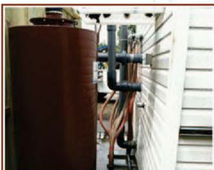
Groundwater Treatment Systems
