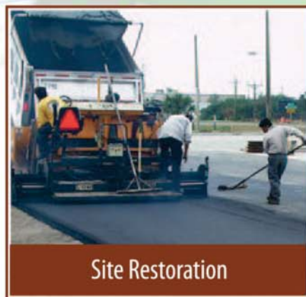
Groundwater Treatment Systems
