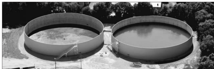
EMERALD COAST UTILITIES AUTHORITY TWO 5.0 MG STORMWATER COLLECTION TANKS CONSULTING ENGINEERS: WARRINGTON; JEHL-HALSTEAD, INC.
