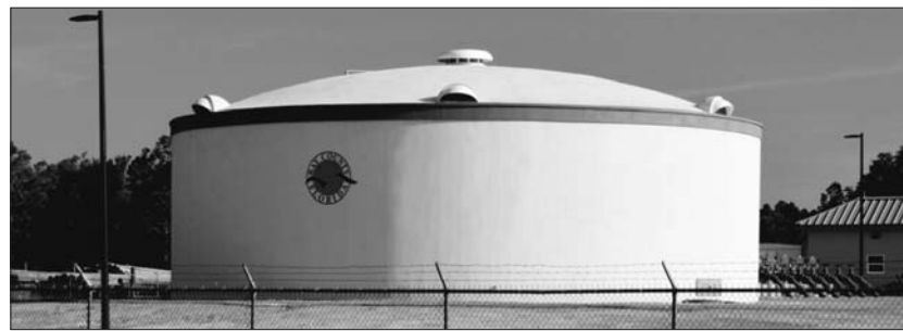
BAY COUNTY - SOUTHPORT 0.5 MG WATER STORAGE TANK CONSULTING ENGINEERS: PANHANDLE ENGINEERING, INC.
